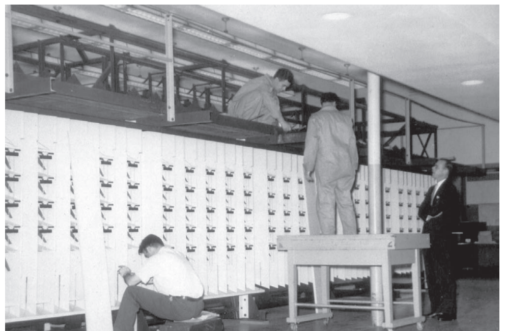
Technicians install the TRANSORMA on January 24, 1957. Operators sat above the mail slots in the area yet to be assembled. Courtesy Silver Spring Post Office.
